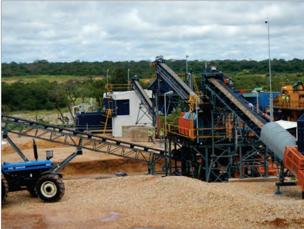
XRT Plant, with scrubber in foreground and the final recovery building in the background
