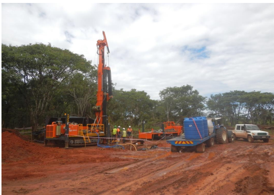
New Hanjin D&B drilling rig in operation at Lulo during the June half
