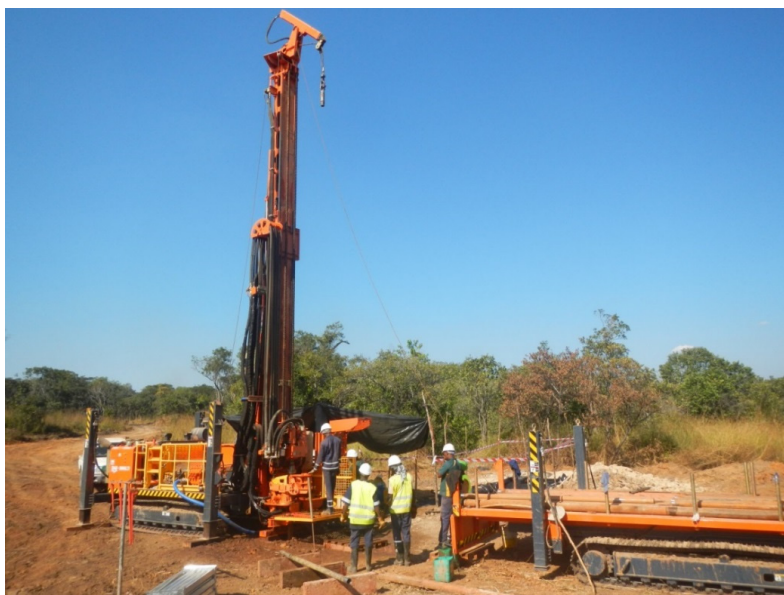
Figure 2: Drilling at the L14 kimberlite discovery at Lulo with the Hanjin D&B35 rig
