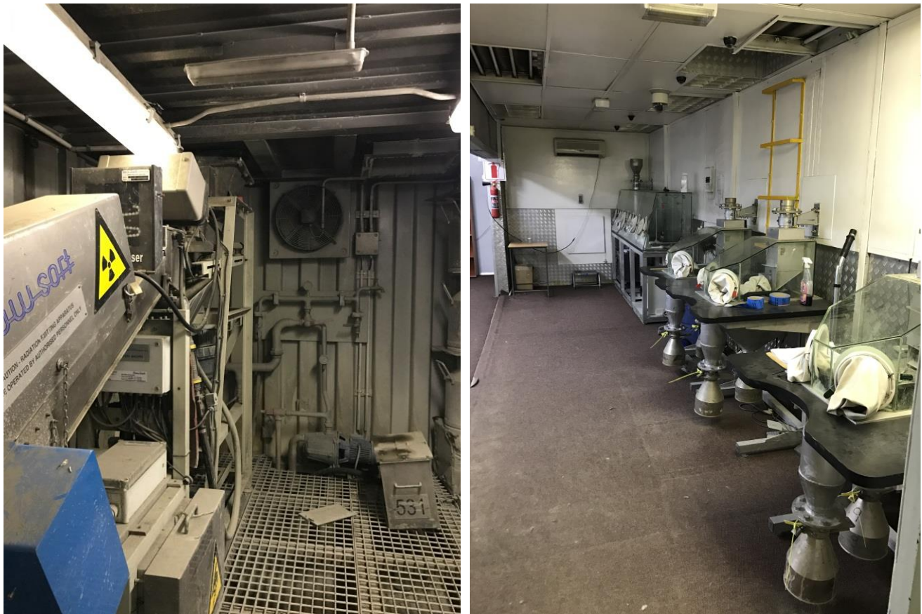
Figure 4: Existing flow sort and recovery rooms at the Mothae kimberlite project
