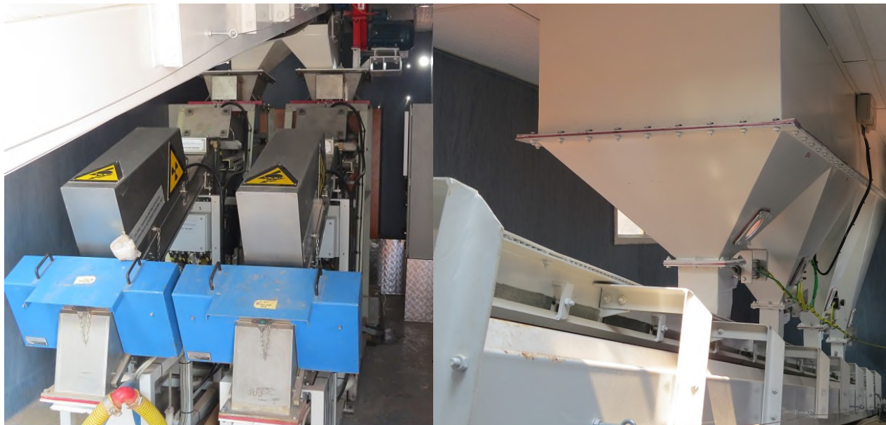
Figure 2: New double pass Flowsort x-ray machines installed at the 150 tph Lulo diamond plant to improve capacity and efficiency of diamond recoveries
