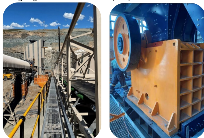
New by-pass conveyor (left) constructed and primary jaw crusher (right) installed as part of the expansion project
