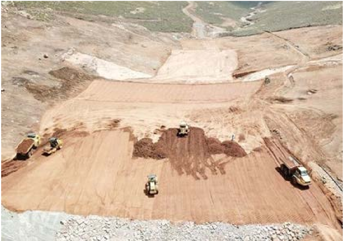
Figure 4: Construction of the wall for the 500,000m 3 water dam at Mothae during the Quarter
